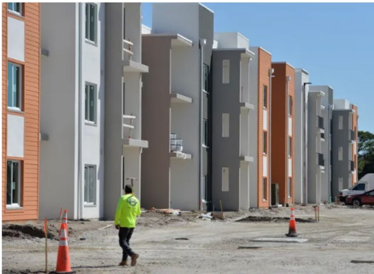
The Sarasota Housing Authority is nearing completion on Cypress Square, a three-building, affordable housing project consisting of 84 units and a clubhouse in the 1600 block of 21st Street in Sarasota. Mike Lang
