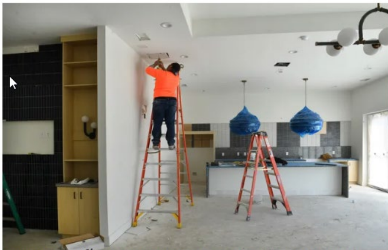
Construction workers are putting the finishing touches on the club house at Cypress Square. The Sarasota Housing Authority is nearing completion on Cypress Square, a three-building, an affordable housing project consisting of 84 units and a clubhouse in the 1600 block of 21st in Sarasota. Mike Lang
