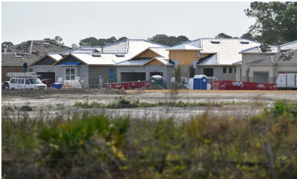
New homes under construction along West Villages Parkway in North Port. Soon, developers in Sarasota County no longer may be required to include affordable housing in their plans. Mike Lang/Herald-Tribune
