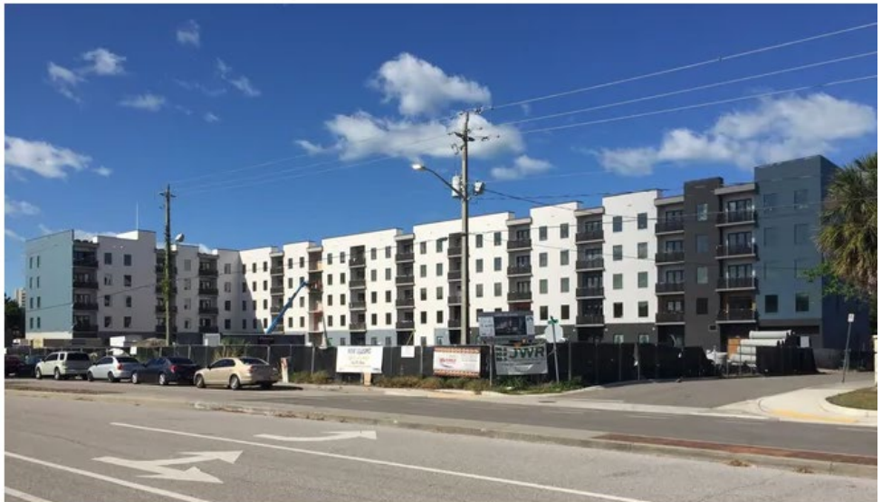
Lofts on Lemon, at 851 N. Lemon Ave. in Sarasota, is expected to be finished later this year. The complex consists of 76 affordable housing units for families earning up to 60% of the area median income, and 52 units for families earning up to 100%. The project was funded by a variety of stakeholders, including the Florida Housing Finance Corporation, the city of Sarasota, the Charles & Margery Barancik Foundation, the Community Foundation of Sarasota County, Bank of America, Freddie Mac, Walker & Dunlop, the Sarasota Housing Authority and the U.S. Department of Housing & Urban Development. Mike Lang / Herald-Tribune
